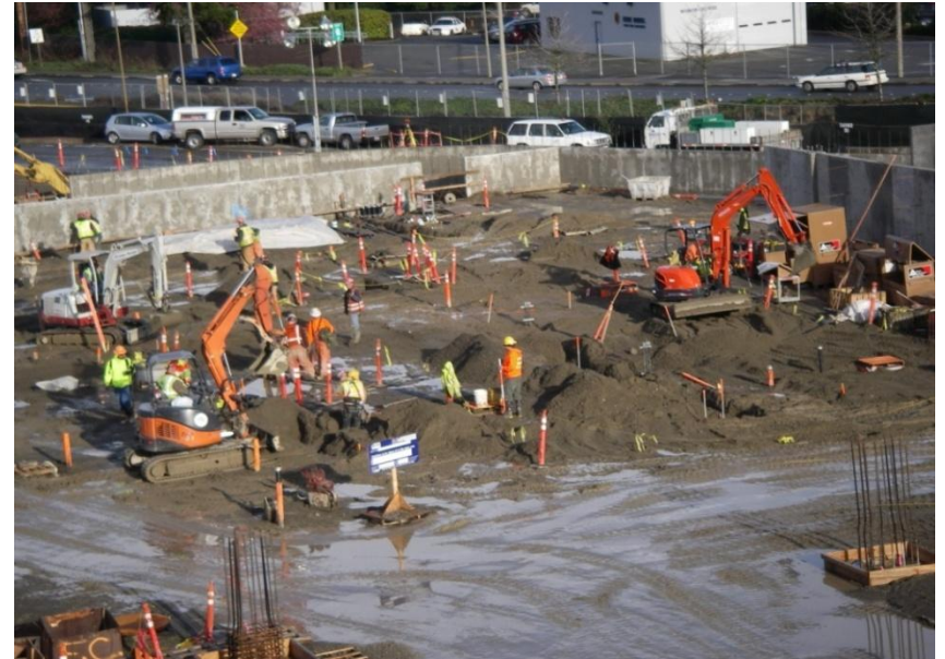
QTA 1: Underground utilities at fueling islands
